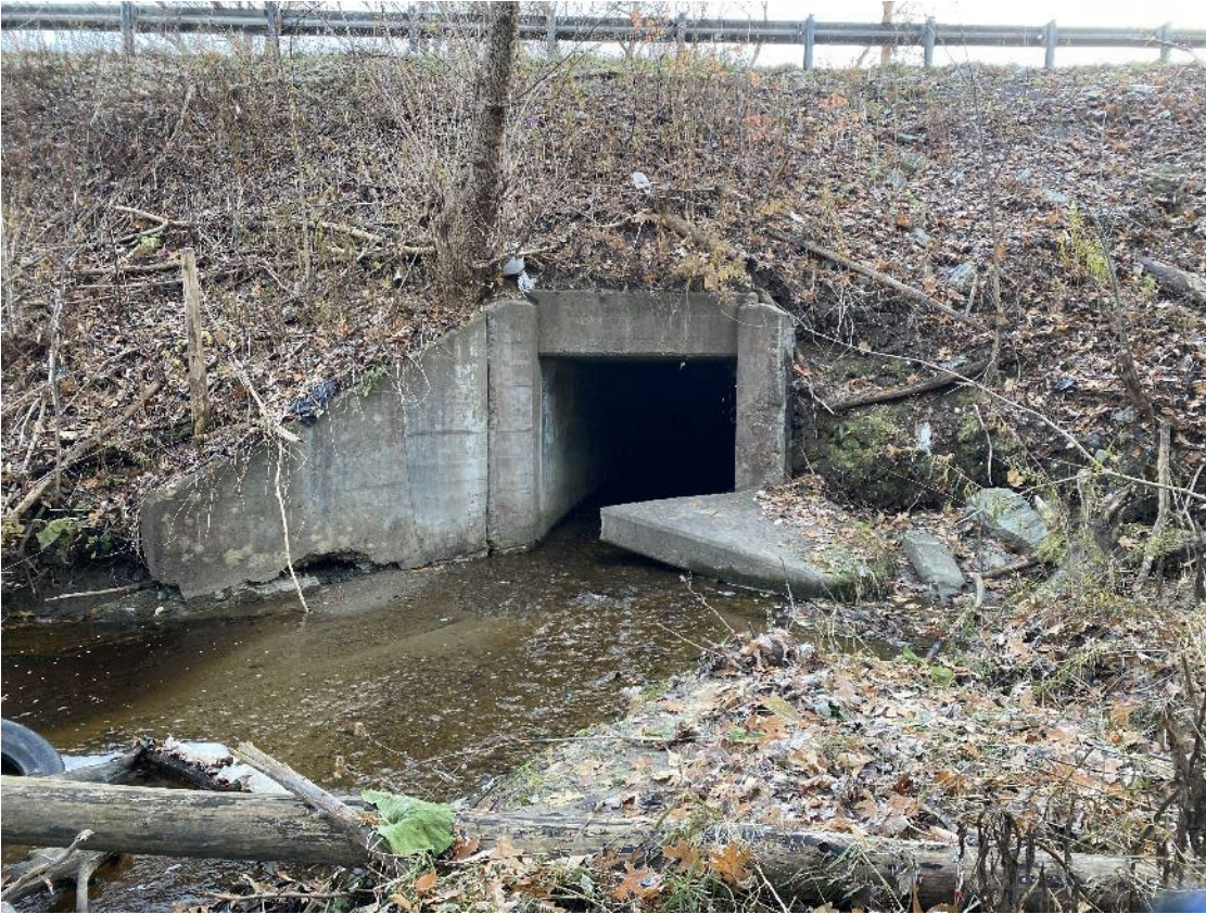
Outlet of box culvert, failed southwest wingwall (Inspection photo 2021)
