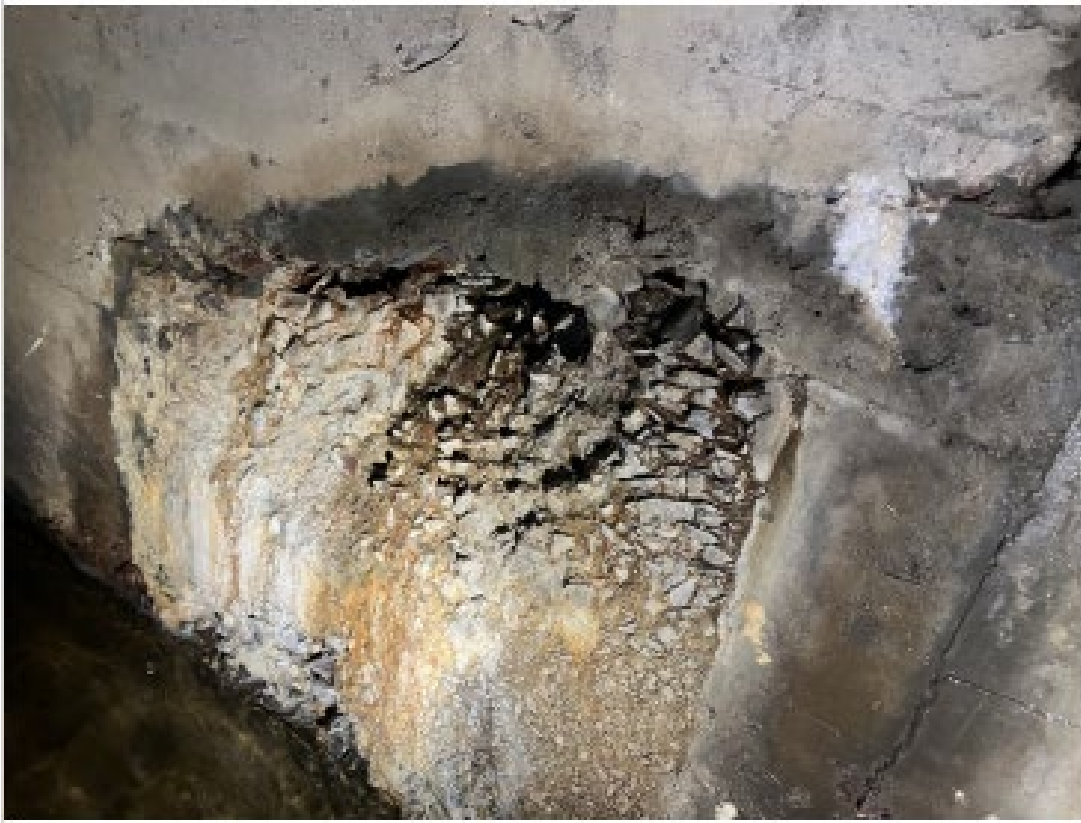
Spalling on Southern Side of culvert upstream end (Inspection photo 11/28/2022)
