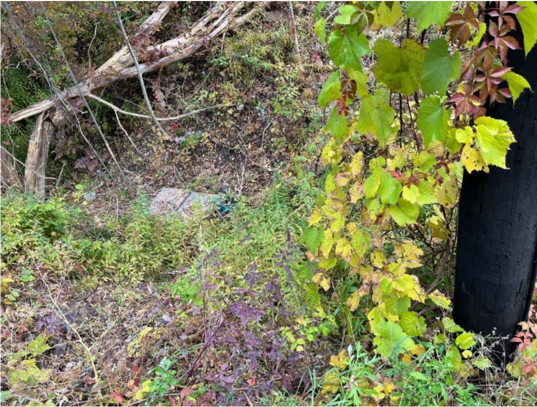
Drop Inlet into structure in median of VT Route 2A and NEC RR
