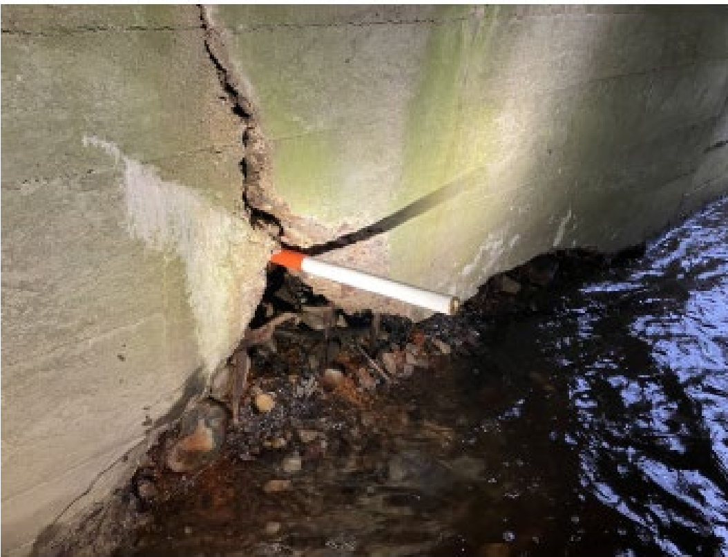
3 feet of backfill sediment loss in spalled area on downstream end southern side (Inspection photo 11/28/2022)
