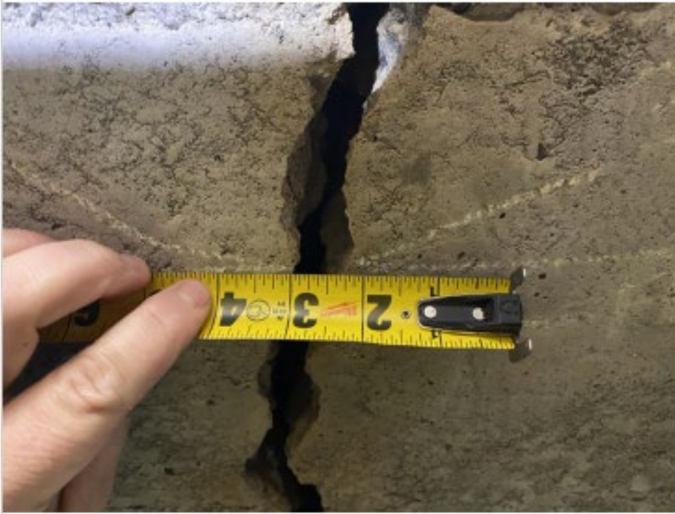
Full Perimeter Crack Below Roadway measuring ~3/4" Wide (Inspection photo 11/28/2022)
