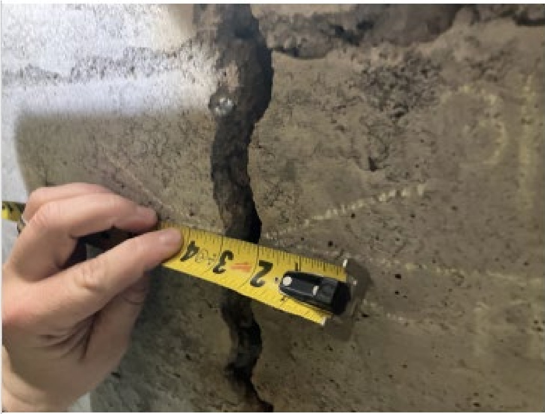
7/8 in crack near downstream end, southern side (Inspection photo 11/28/2022)
