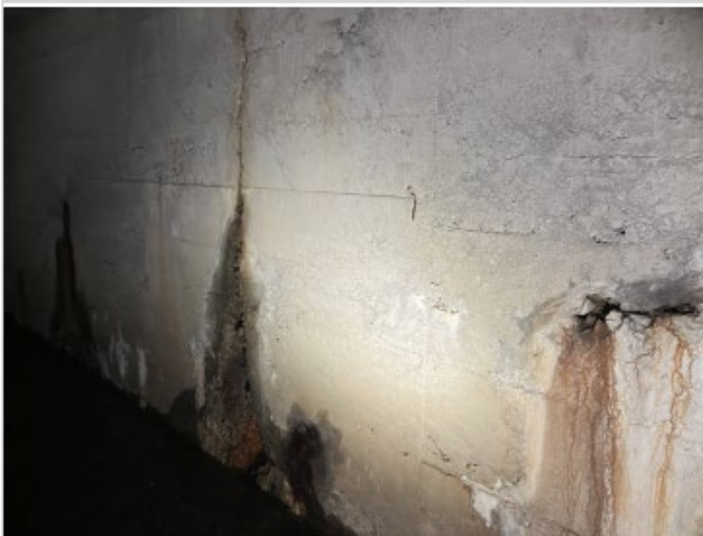
Spalling and cracking on Southern Side of Culvert between downstream and Midspan (Inspection photo 11/28/2022)
