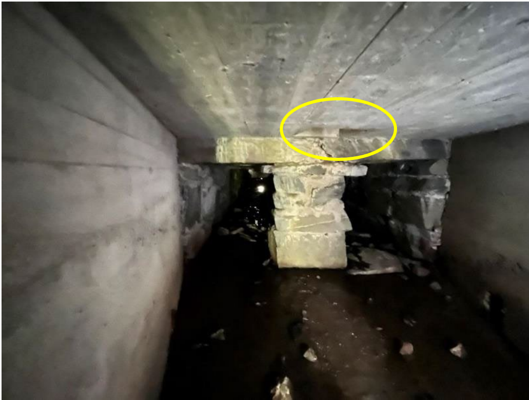
Drop inlet from median between NEC RR and VT Route 2A visible at connection point (circled in yellow)
