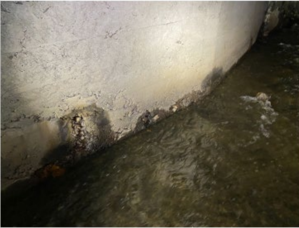
Northern Box Walls Leakage / Spalling (Inspection photo 11/28/2022)
