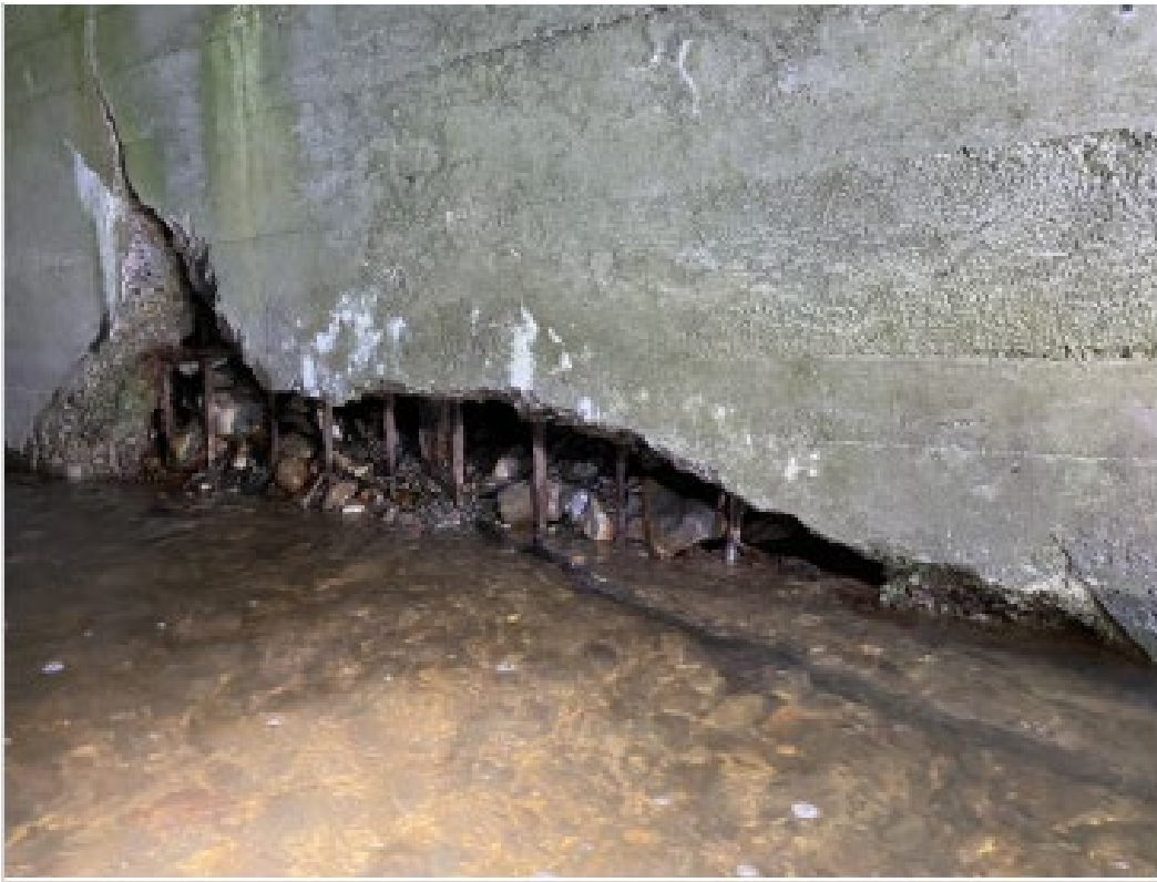
Severe Spalling with Severed Steel Reinforcing along Southern Box Wall (Inspection photo 11/28/2022)
