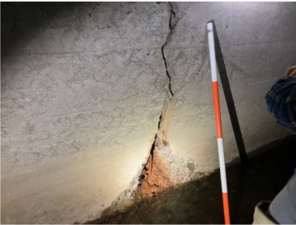
Spalling and full perimeter crack on northern side of culvert between downstream and Midspan (Inspection photo 11/28/2022)
