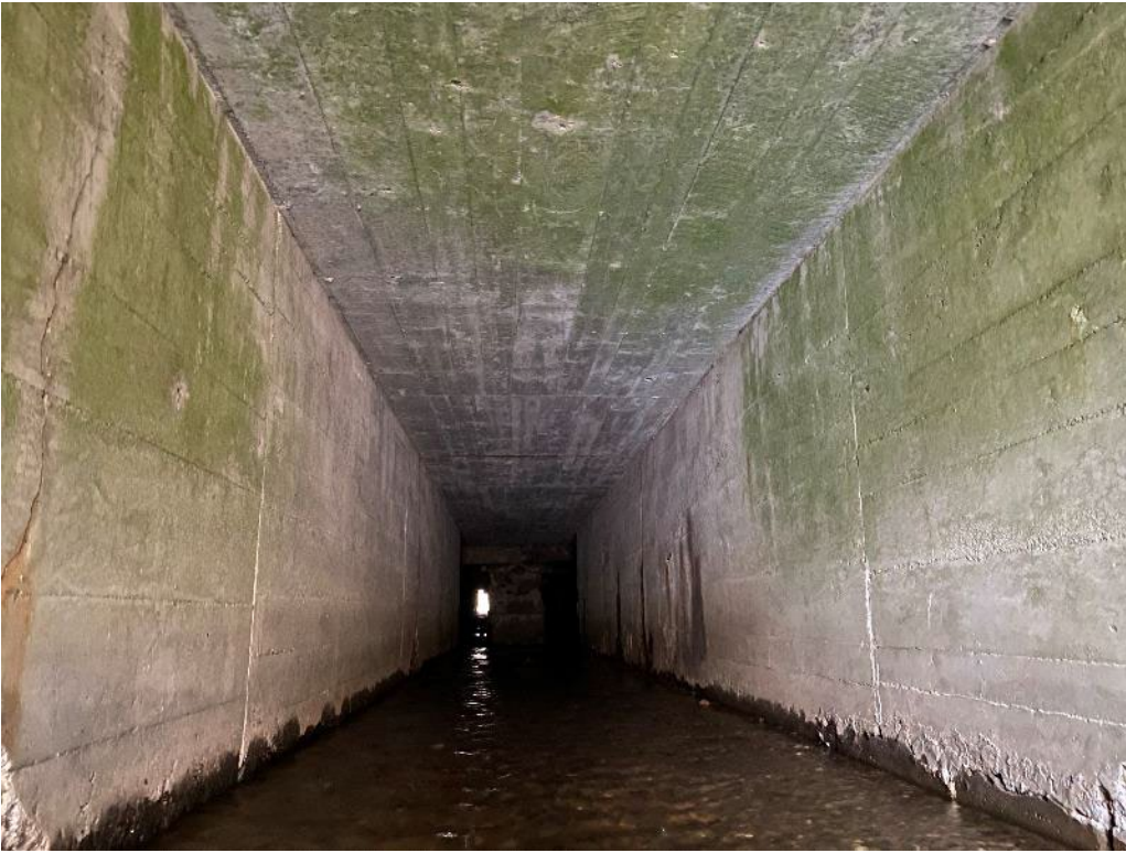
Facing upstream through culvert from downstream with full perimeter cracks over spalled areas (Inspection photo 11/28/2022)
