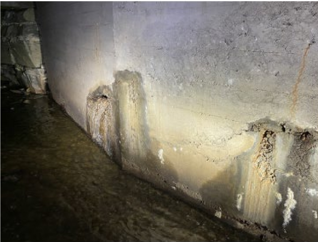
Southern Box Walls Leakage / Spalling (Inspection photo 11/28/2022)
