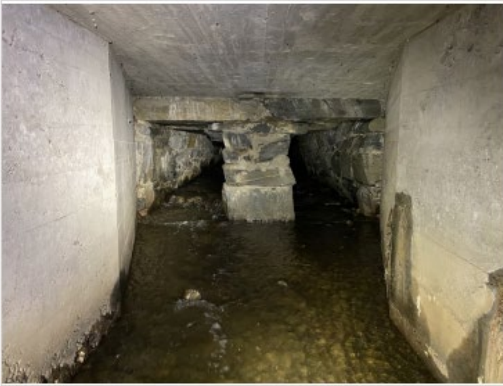
Upstream End of Box Culvert, connection point of laid up stone box culvert section underneath the New England Central Railroad (Inspection photo 11/28/2022)
